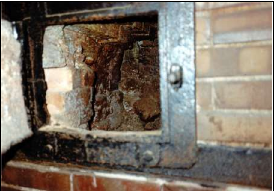
Photograph 9: Right-hand gasifier: coke-loading door.
