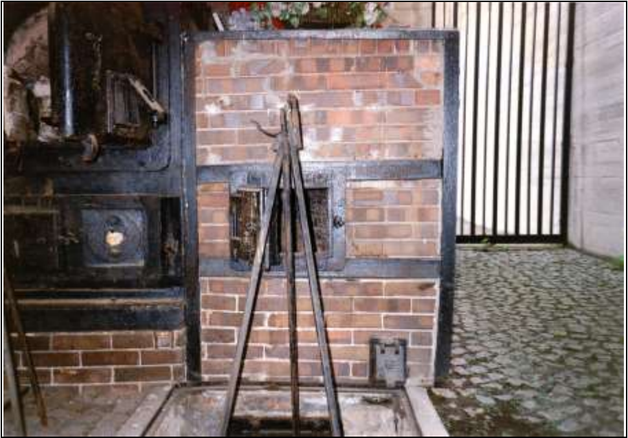
Photograph 8: The furnace's right-hand gasifier with coke-loading door and the gasifier's primary air intake.
