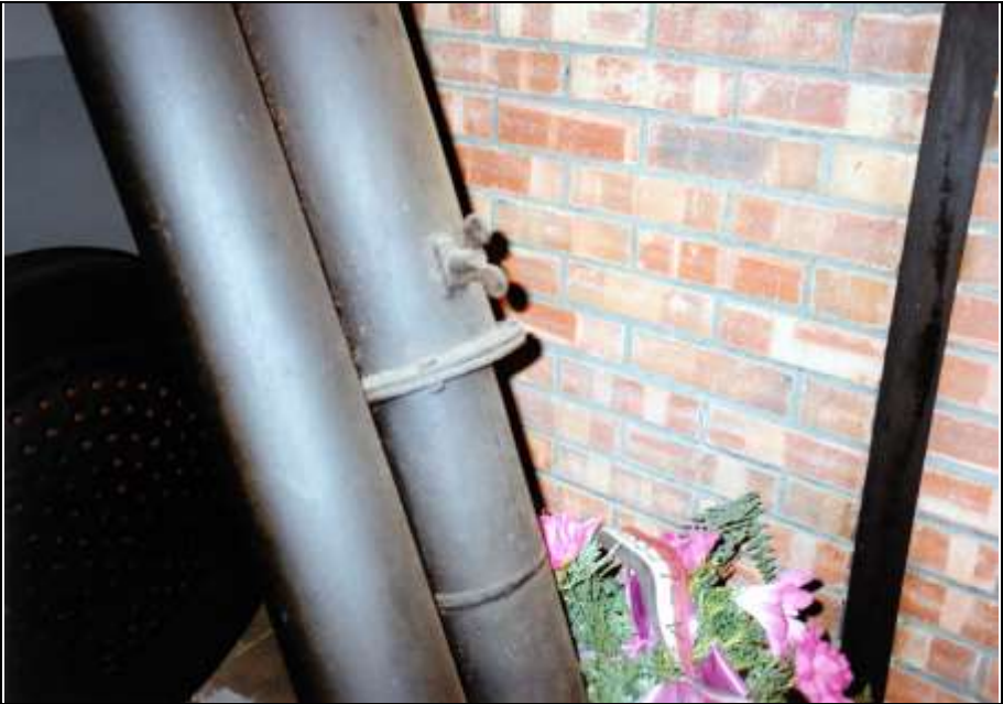
Photograph 194: Tube from the combustion-air blowers to the furnaces; butterfly valve in the right-hand tube for regulating the air flow.
