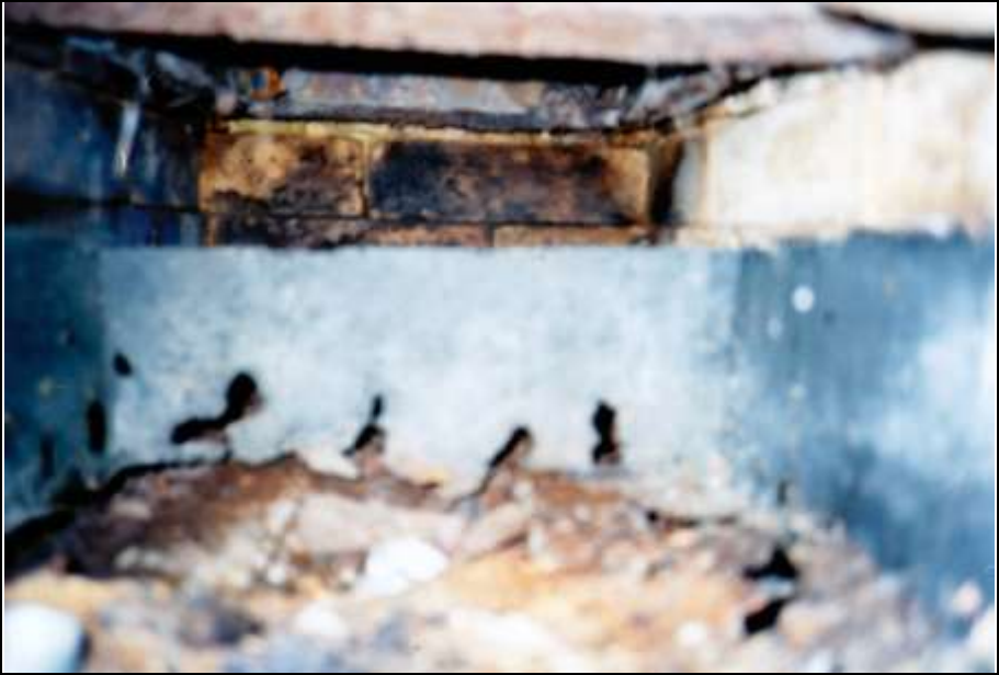
Photograph 355: as above; inside of the ash chamber seen through its rear service door, with the corroded iron ash container.
