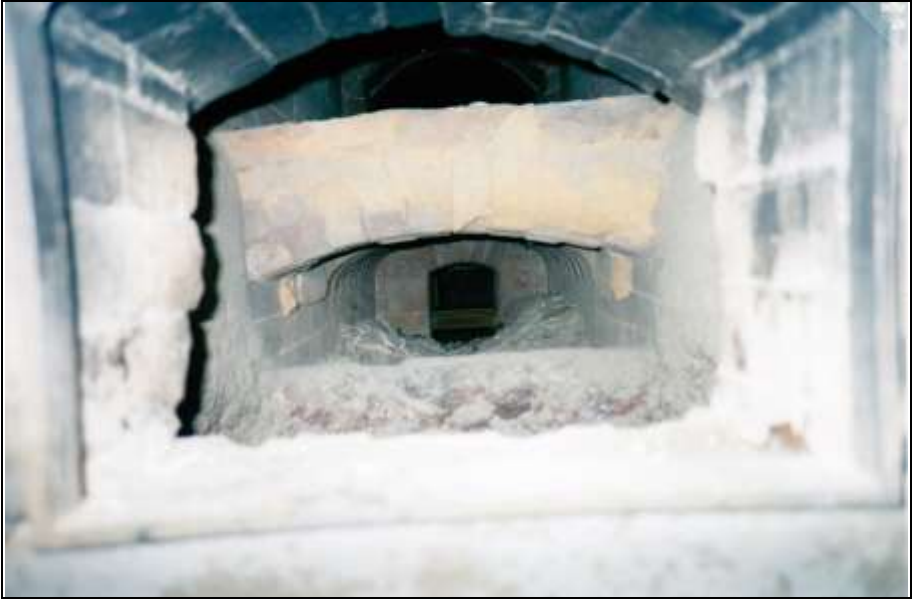
Photograph 313: Inside of a furnace seen from the gasifier's coke-loading door. Foreground: the gasifier; behind it: the ash chamber with the ash doors in the background; above that: the muffle's fireclay grate; top: the muffle.
