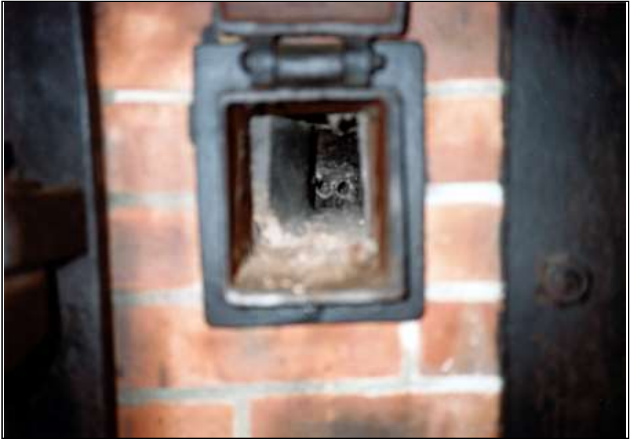
Photograph 149: as above, the muffle's combustion-air-supply channel.
