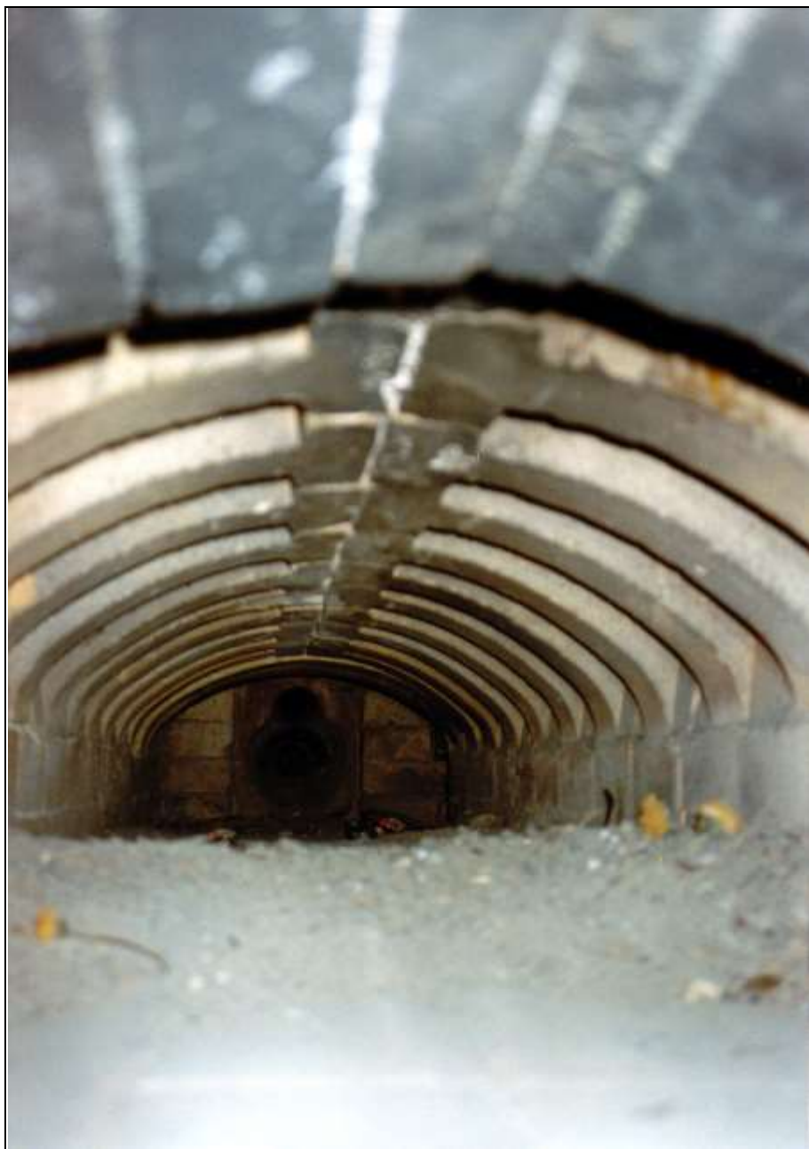
Photograph 323: Ash chamber; top: the underside of the muffle's refractory grate; background: the auxiliary burner's nozzle.
