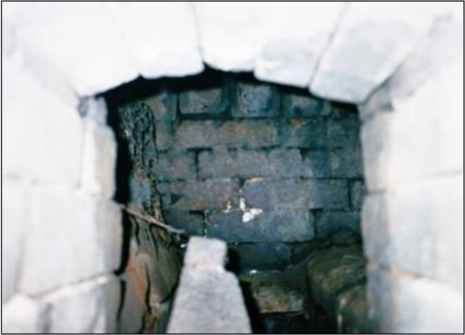
Photograph 281: as above. View into the auxiliary gasifier. Background: the wall of the muffle's ash chamber. Foreground: the end of an iron bar from the auxiliary hearth grate.
