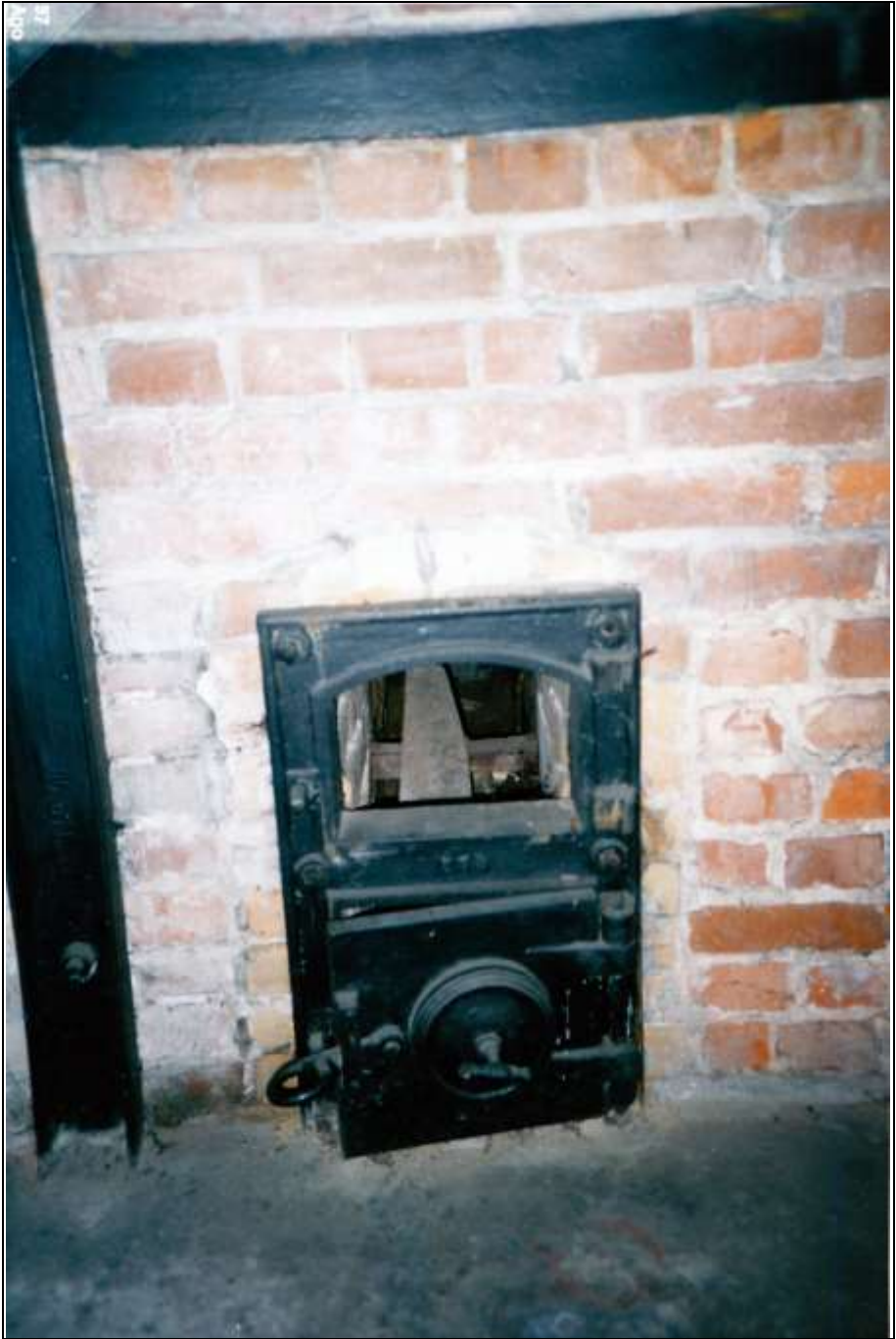
Photograph 280: Left-hand furnace; doors of the auxiliary gasifier.
