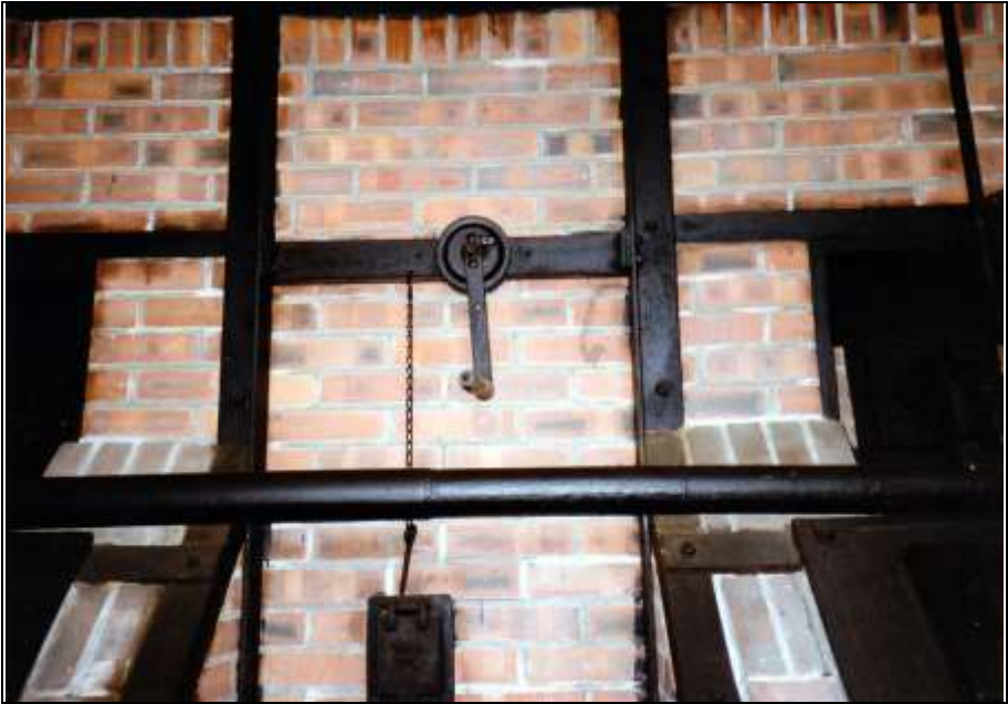
Photograph 168: as above, central muffle. Crank operating the smoke-duct damper (top) and the door to the muffle's rear combustion-air channel (bottom).
