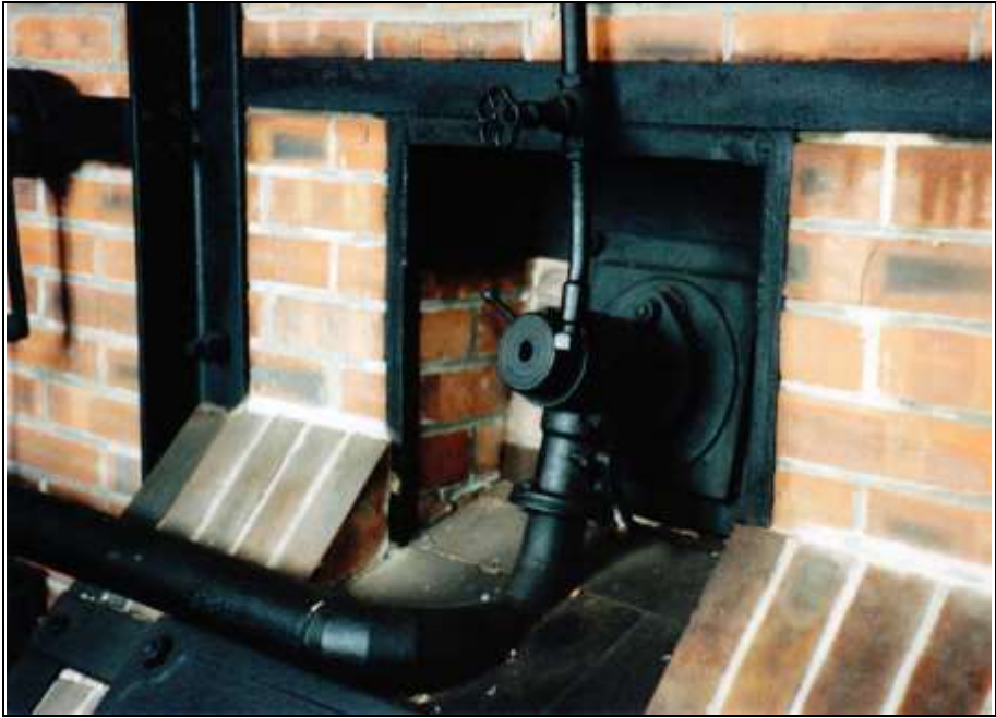
Photograph 204: as above, rear view, naphtha burner of the left-hand muffle; connected to the naphtha burner are from above, the tube feeding oil from the naphtha tank, and from below, the tube from the combustion-air blower.
