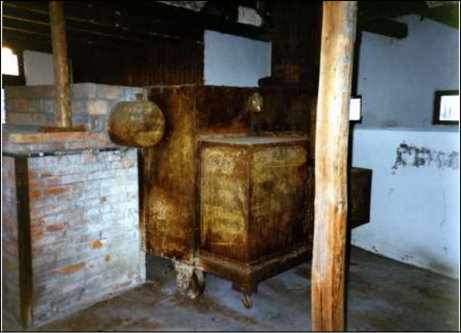
Photograph 45: Rear of the furnace, right-hand side. At the top of the gasifier, the rear part of the original oil tank protrudes, which was walled-in. The furnace's original body is mounted on metal wheels.
