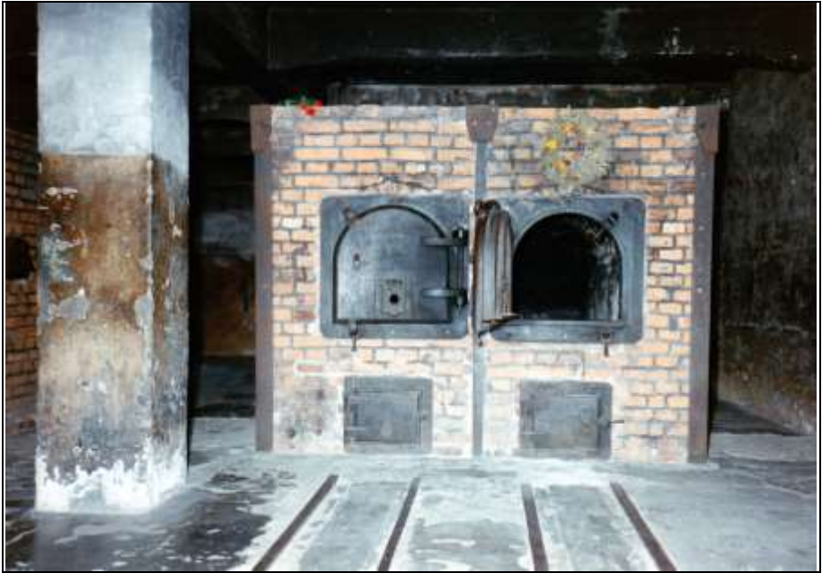
Photograph 90: Furnace No. 2. The refabrication omitted the transverse anchor bars and the combustion-air-intake channels next to the muffle doors; in addition, the muffle doors were reversed. Compare Photo 51.
