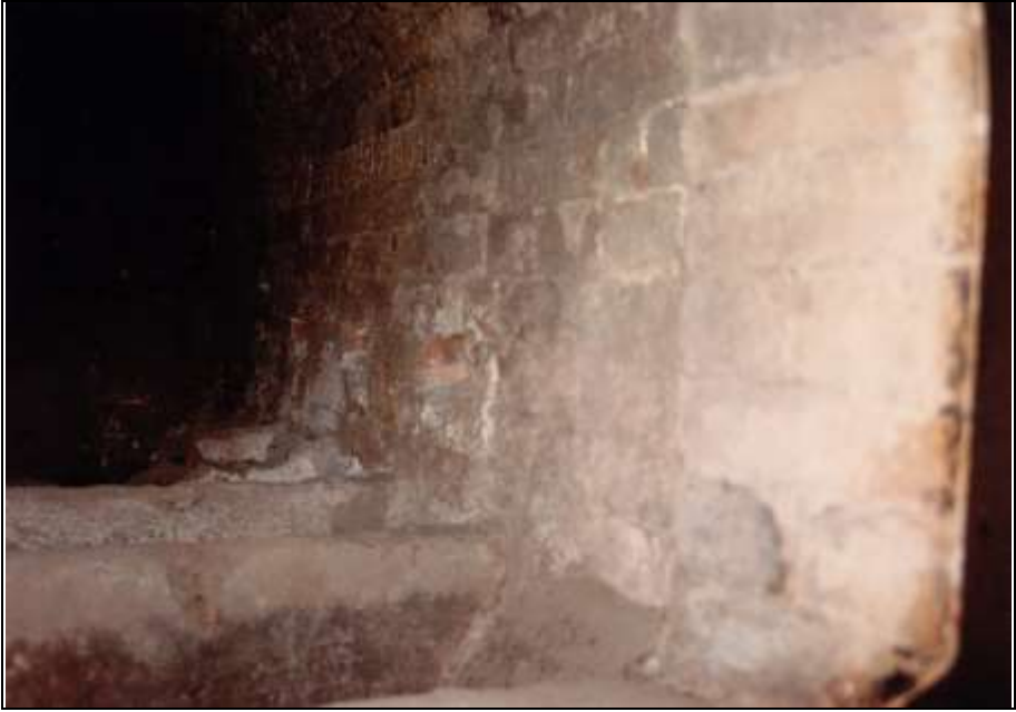
Photograph 147: as above, right-hand square openings of the combustion-air feed. Bottom: muffle grate.
