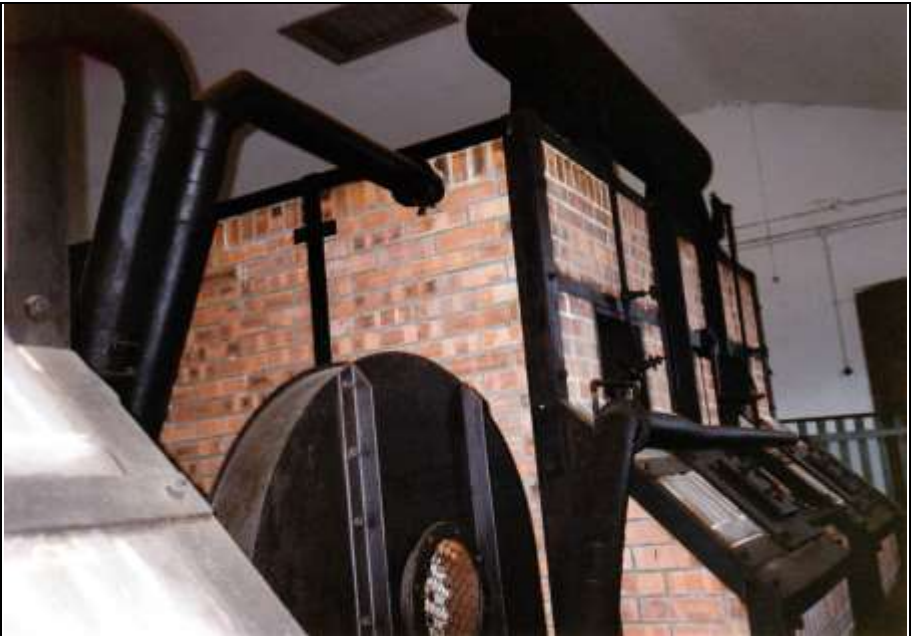
Photograph 198: as above, left-side rear view with tube running into the furnace.
