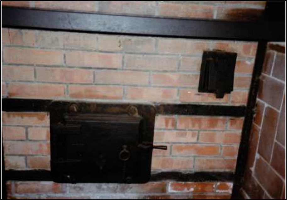
Photograph 165: as above; the gasifier's ash-chamber door (bottom) and the door of the gasifier's combustion-air channel (top right).
