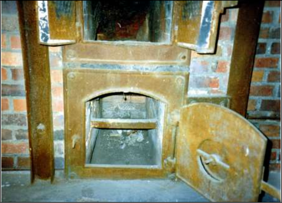
Photograph 262: Ash-chamber door of the main gasifier.
