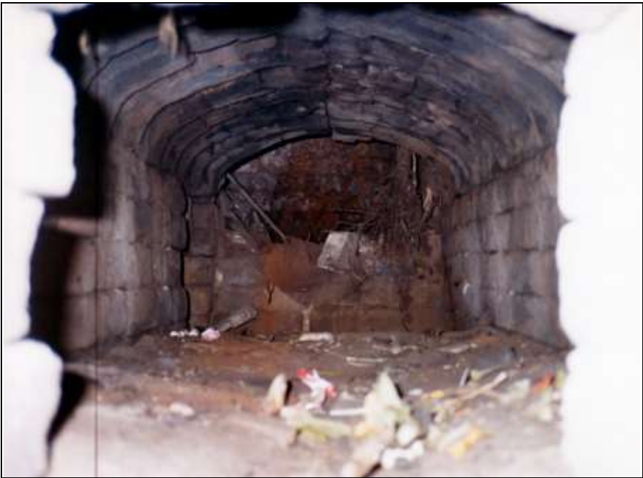
Photograph 273: The ash chamber of the left-hand muffle. Top: underside of the muffle's grate bars. On the left wall in the rear: opening connecting it with the auxiliary hearth. All the way at the back: the gasifier's pit.
