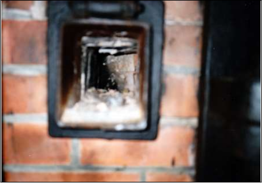
Photograph 151: as above, the muffle's combustion-air-supply channel.
