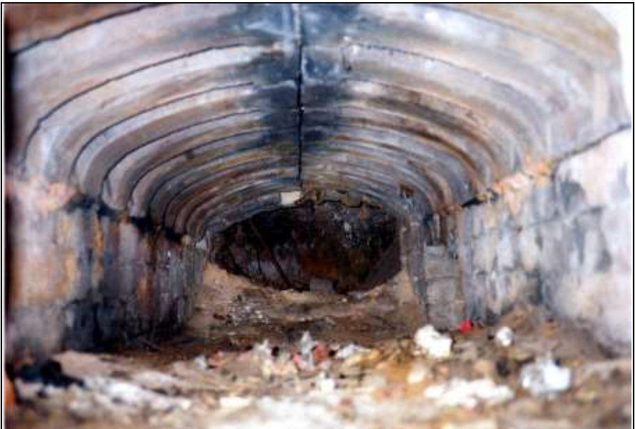
Photograph 275: as above, ash chamber.
