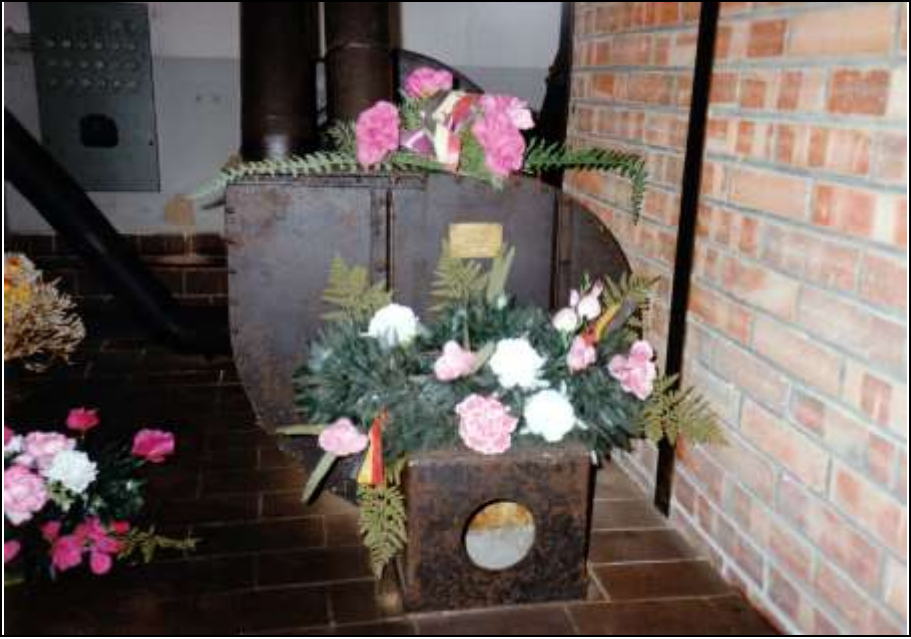
Photograph 189: The furnaces' combustion-air blower, front view; the left tube feeds the furnace fueled with either coke or naphtha, the right tube the coke-fired one (see Photo 188).
