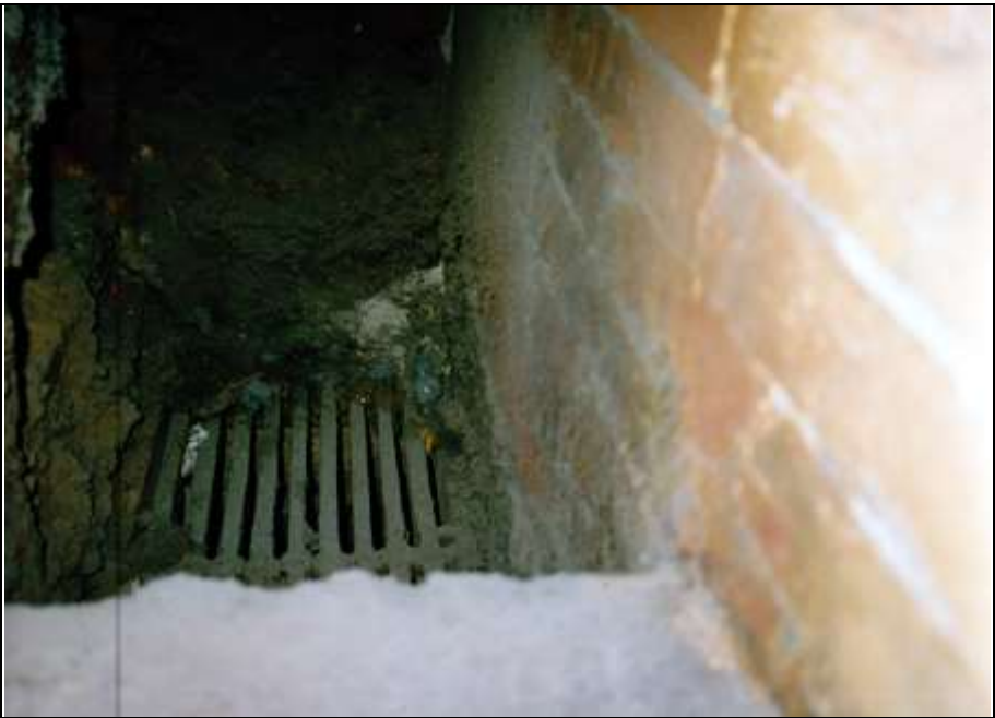
Photograph 263: View into the main gasifiers.
