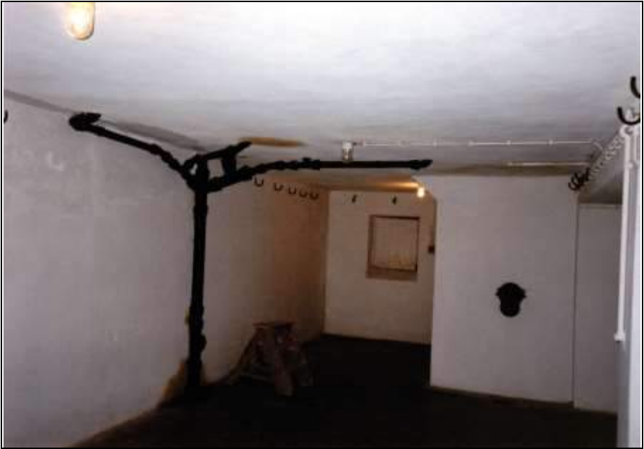
Photograph 211: as above; on the back wall, on the right, the manual controls for operating the freight elevator.
