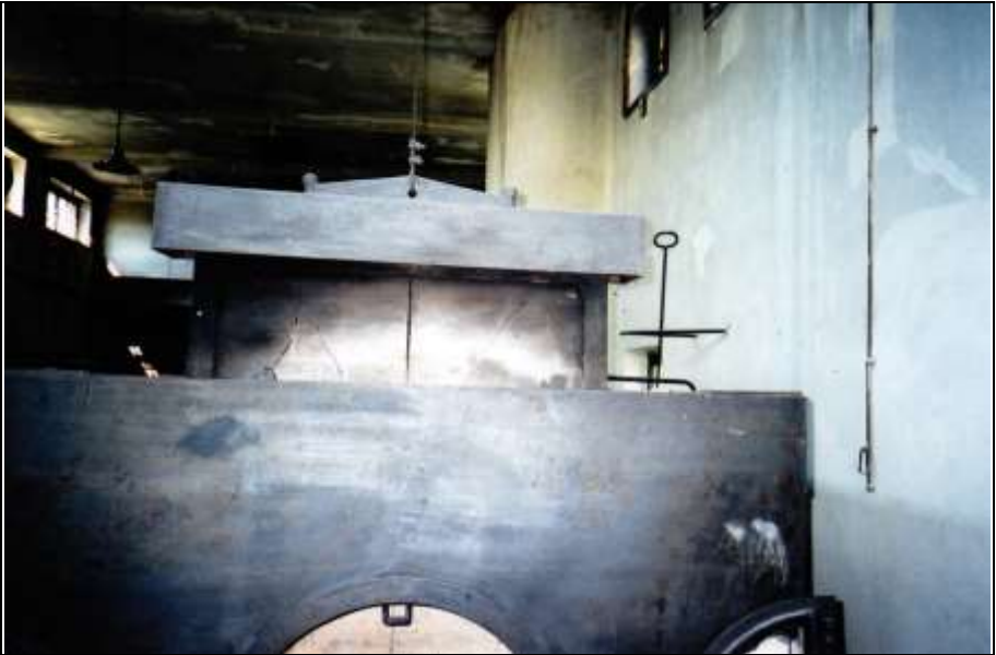
Photograph 359: Closing damper of the right-hand furnace of the rear pair of furnaces.
