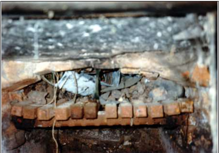
Photograph 174: as above; view into the gasifier's ash chamber with the grate.
