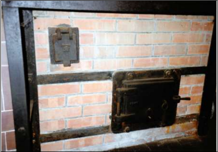
Photograph 173: as above, right-hand muffle. The gasifier's ash-chamber door (bottom) and the door of the gasifier's combustion-air channel (top left).
