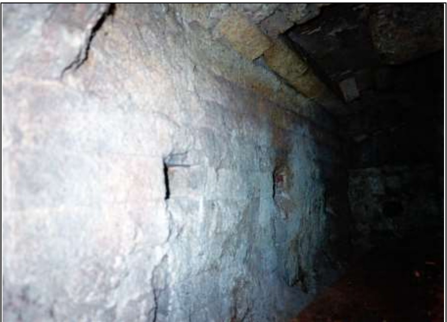
Photograph 241; as above, close-up of combustion-air-supply holes.
