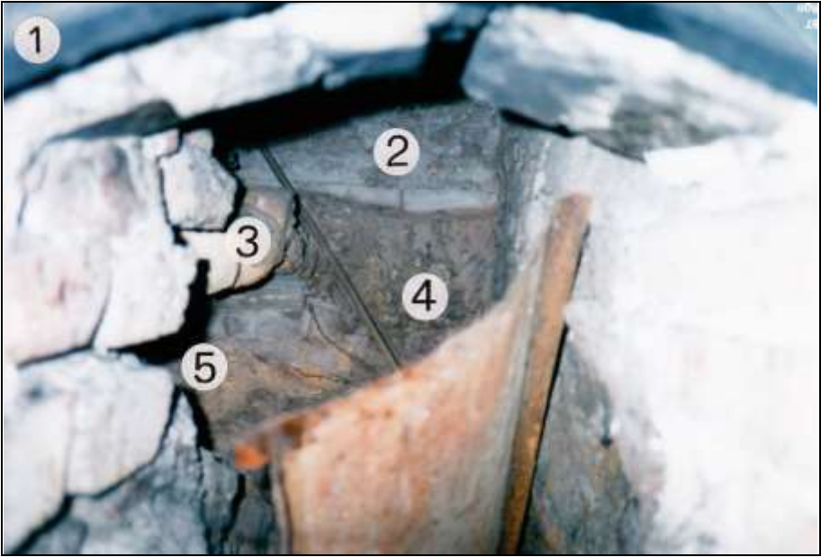
Photograph 278: as above, seen through the coke-loading door. 1: door frame; 2: muffle; 3: muffle grate; 4: gasifier pit; 5: ash chamber.
