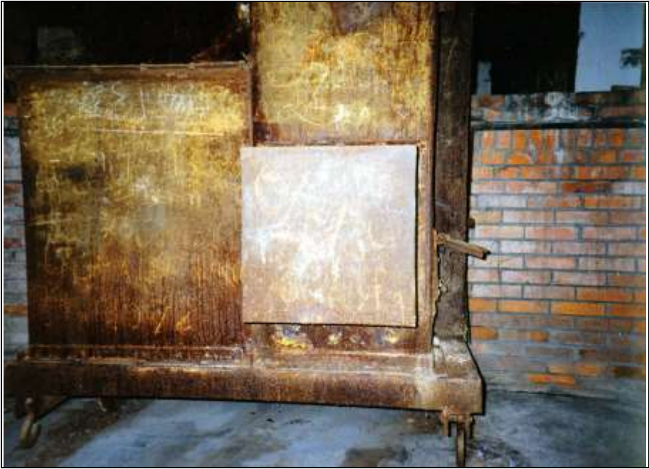
Photograph 47: Rear view of the furnace; base of the chimney with an open service door at the right-hand side. The square metal sheet welded to the chimney's bottom closes the opening for the original forced-draft blower.
