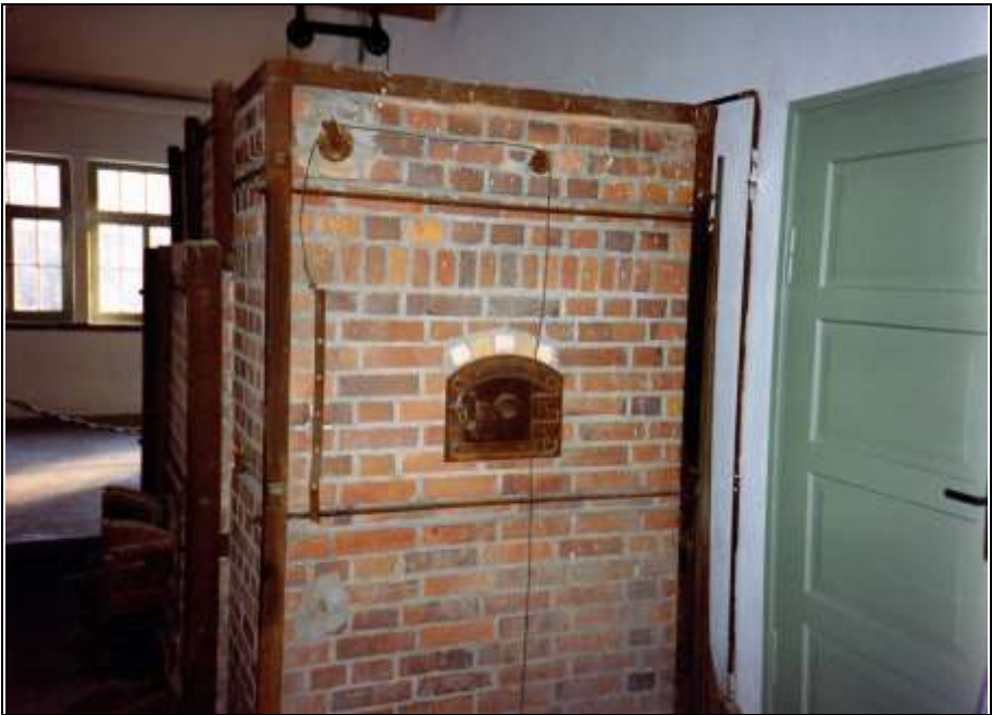
Photograph 259: Rear view of the first furnace; inspection door of the vertical smoke duct. Wire cable and pulleys for operating the smoke-duct damper, visible in Photo 258 on the floor at the bottom of the furnace.
