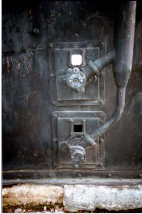
Photograph 333c: rear view, main (top) and auxiliary burner (bottom)
