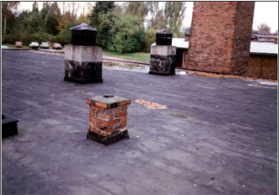
Photograph 104: Roof of Crematorium I: The two ventilation chimneys of the cremation furnaces (black and grey).
