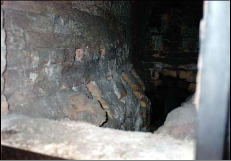
Photograph 131: as above; in the left-hand wall four openings of combustion-air channel are visible; below this the remnants of the muffle-grate bars and the walls slanted toward the ash chamber; in the back at the bottom is the opening to the gasifier.
